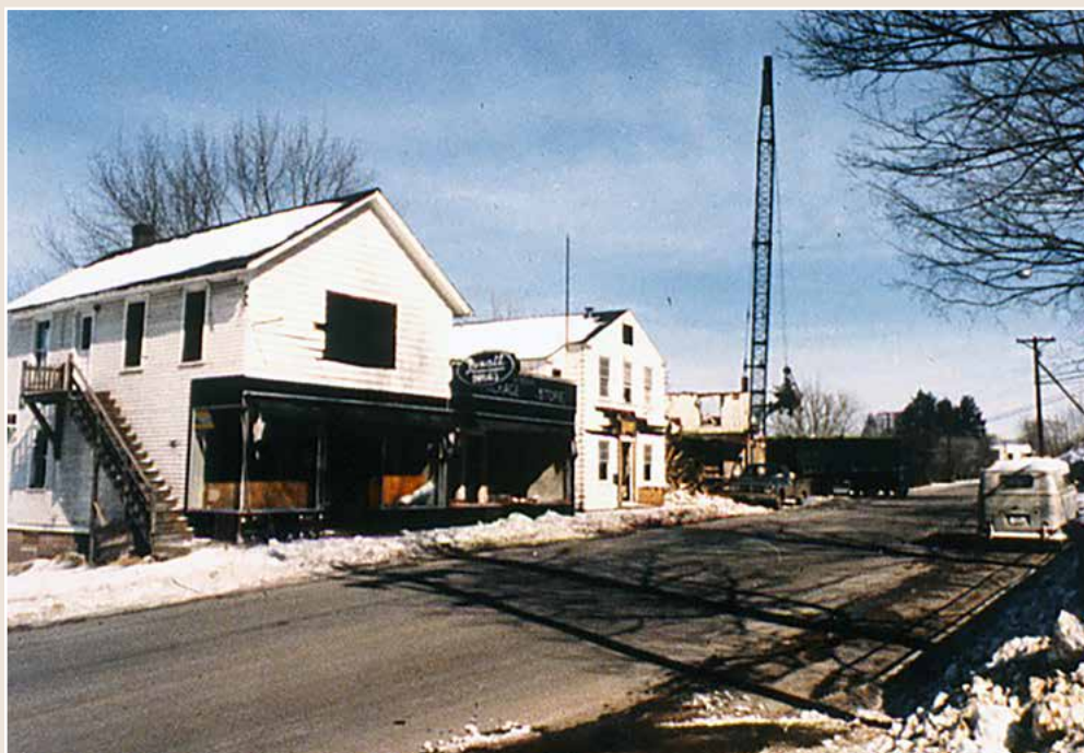
Some of the nicest buildings in the business district started to come down. It was then that townspeople began to have second thoughts about their approval of the project. Photos courtesy of Ken Simon.
